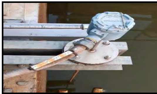
Figure 3.2 Temperature Sensor Location at Central Monitoring Basin
